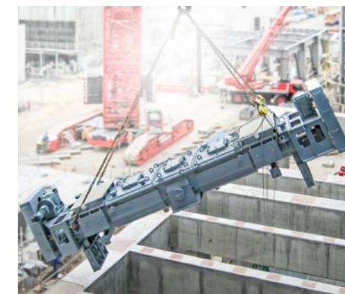
5. Double cooling screw conveyor
